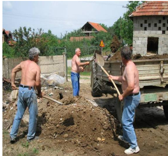
The dirt from the digging is being transported by the rented tractor from the site.
